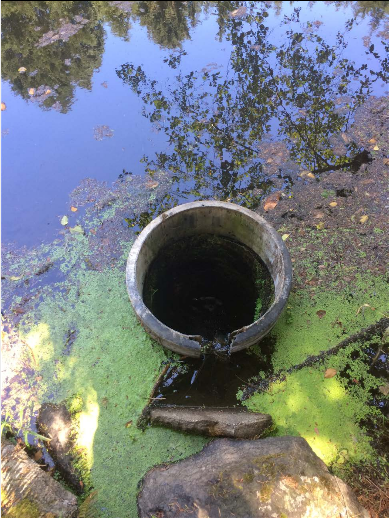
Picture 2: Pond outlet to private culvert (~3-4 foot drop from top of outlet to culvert).
