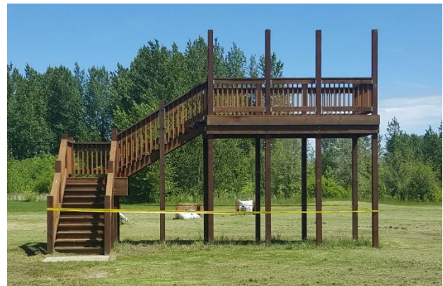
New elevated shooting platform at the EE Wilson Wildlife Area Archery Park
