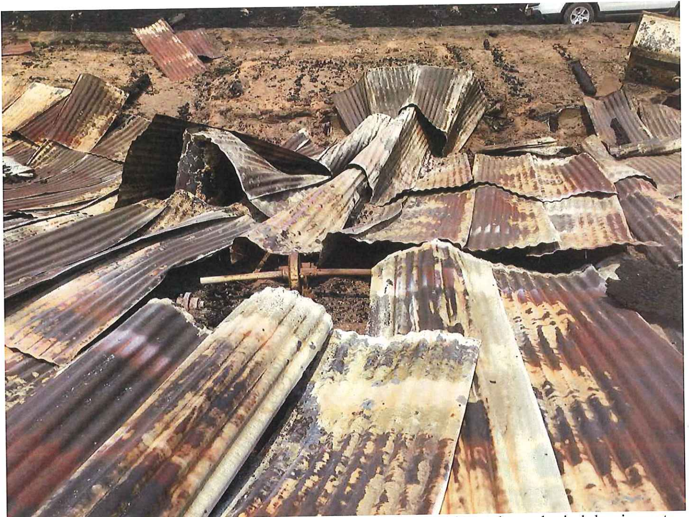
Figure 10. "Harris Ranch Shearing Shed and Corrals." The shearing shed featured a mechanical shearing system (axle pictured in center). It was built at an unknown time after the Harris House, but the worker bunkhouse (pictured below) associated with the shearing shed was constructed out of two railroad cars associated with the Deschutes Railroad that was deconstructed around the 1930s. Facing East.
