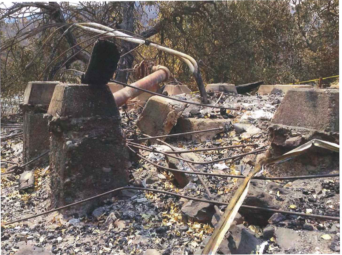
Figure 21. Support pillars are the only intact feature remaining of the water tower. Facing west-northwest.
