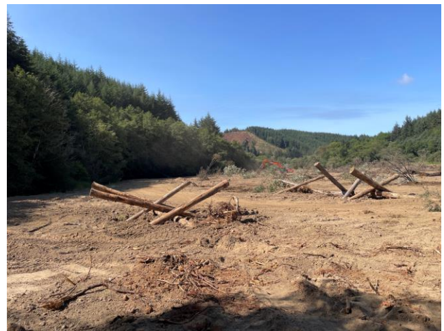
Non-native canary grass was removed, and the area was then planted with willows and log structures were created.
