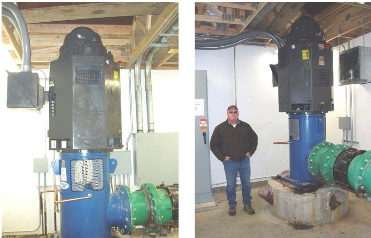
Figure 12. New 500-hp well pump installed at Bonneville Hatchery.
