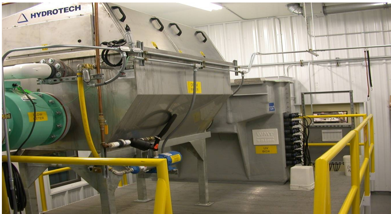
Ultraviolet water disinfection system at Lookingglass Hatchery
