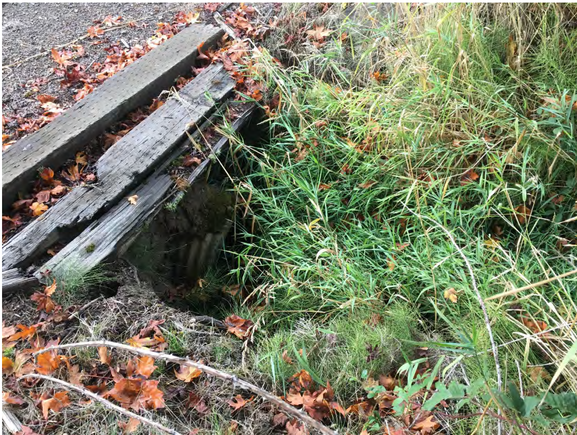
PHOTO 12 October 13, 2017 View of a culvert under SW Scoggins Valley Road that conveys a Scoggins Creek tributary in the Option 3 impact area. There was no flow at this location during the site reconnaissance, and the culvert appeared to be at least a partial passage barrier
