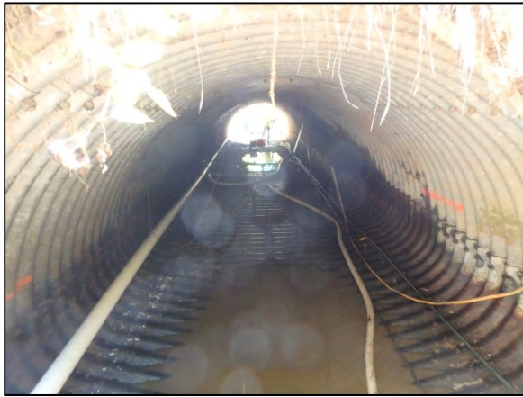
Potter Creek Culvert pre-treatment (left), post-treatment (right)
